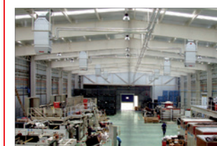
TopVent® MK units provide the right climate in a production plant for automotive components.
