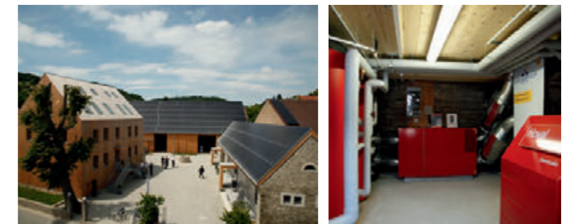
Model ecological solution in a complex with residential and commercial buildings: A heat network provides heat from a ground water heat pump, comfort ventilation system with heat and humidity recovery, and photovoltaic system with SmartGrid.
